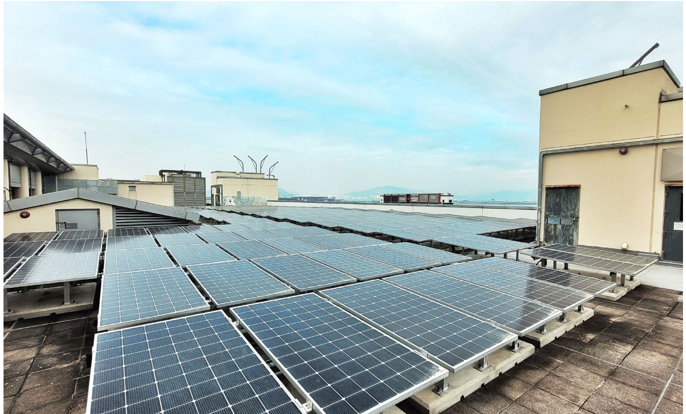
Solar panels have been installed on the rooftop of Cathay City, our headquarter building
